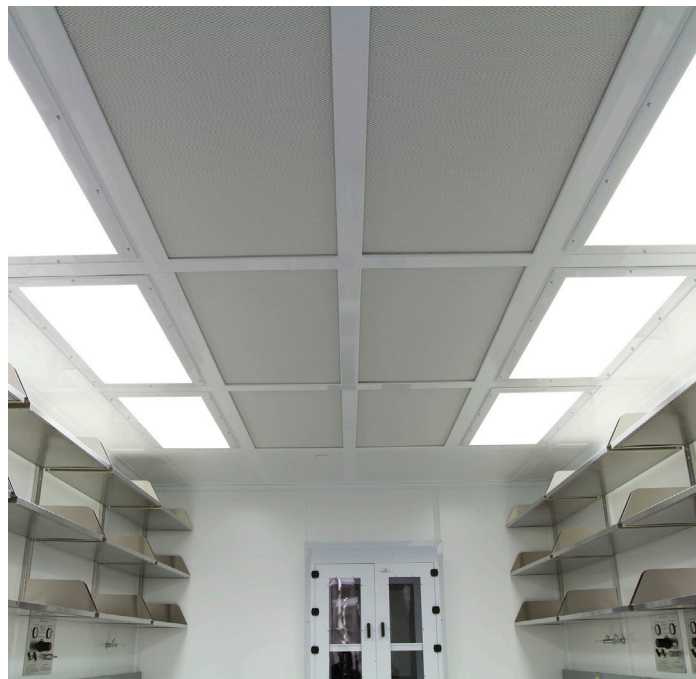
Buffer Area rated ISO 7 with HEPA Filters and SAF fixtures in the ceiling. NOTE: Pass through in center.
